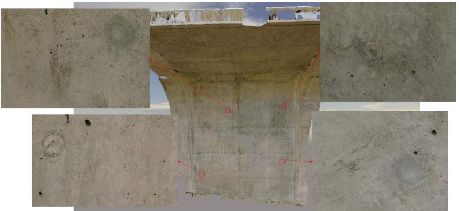
Figure 4.57: Context Capture 3D Mesh Model of Segment P3-3U on the Southbound Bridge
