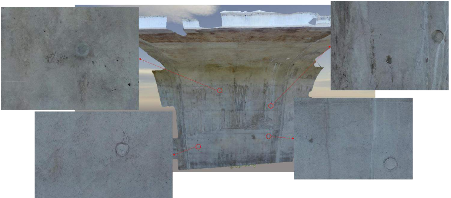
Figure 4.55: Context Capture 3D Mesh Model of Segment P3-3D on the Southbound Bridge
