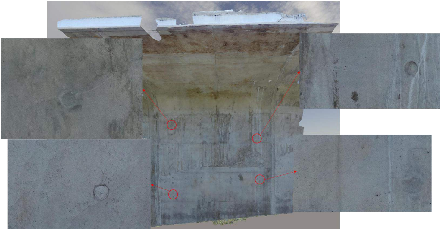
Figure 4.53: Context Capture 3D Mesh Model of Segment P2-3U on the Southbound Bridge
